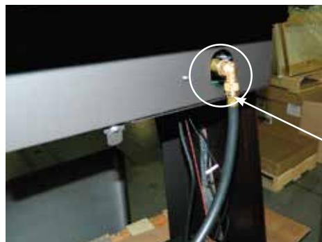
Gas connection @ unit
