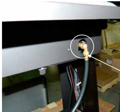
Gas connection @ unit
