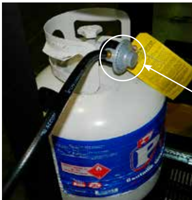
Gas connection @ tank
